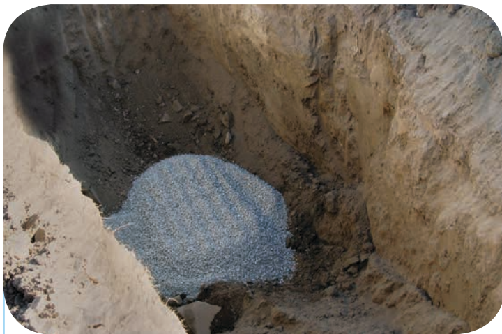
Example of a bentonite topseal installed during the decommissioning of bored well
